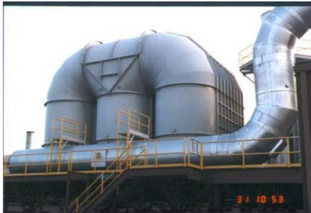
Typical 3 Chamber RTO
